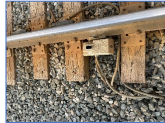
BELOW: Close up of Hot Box Detector
