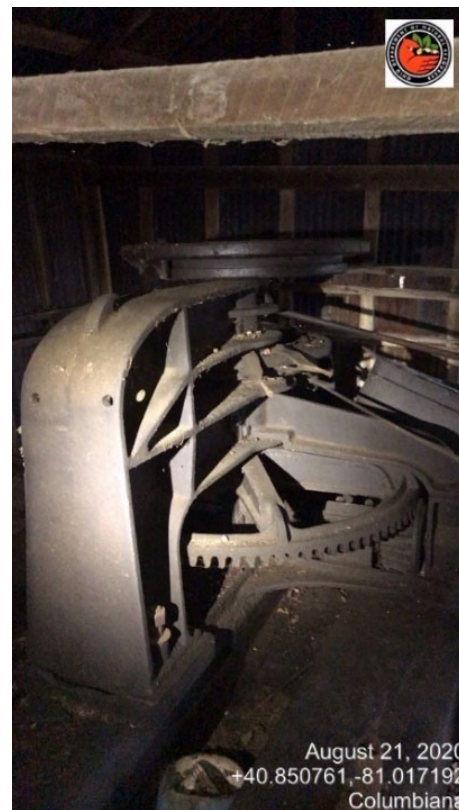
Columbiana #3 Project, Inside Powerhouse
